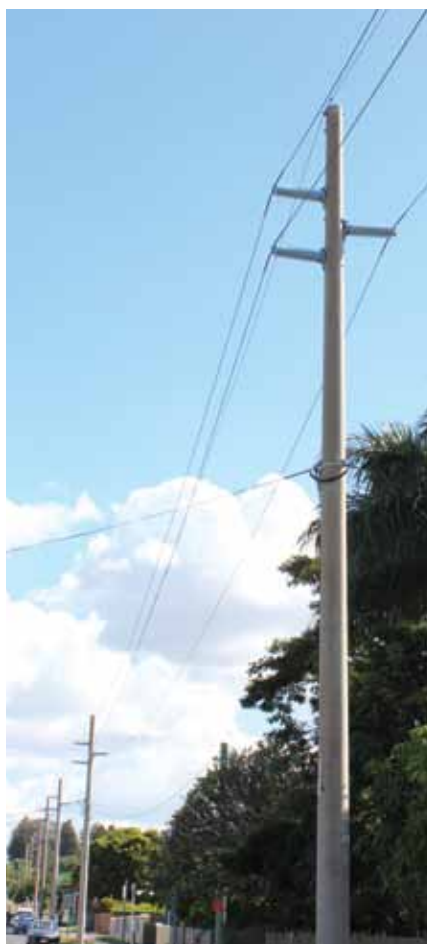
Example of a typical urban 66,000 volt concrete pole powerline
