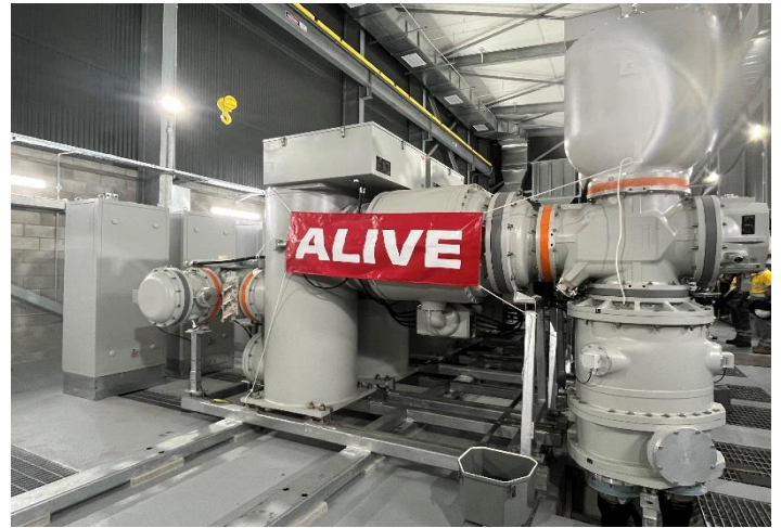
Fig 4 – The Belgian Gardens feeders are connected to the switchgear at the Garbutt substation and energised.
