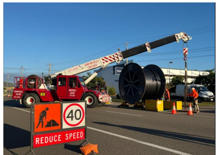
Fig 1 – A franner lifts the 66,000-volt cable drum into position on Dalrymple Road.
