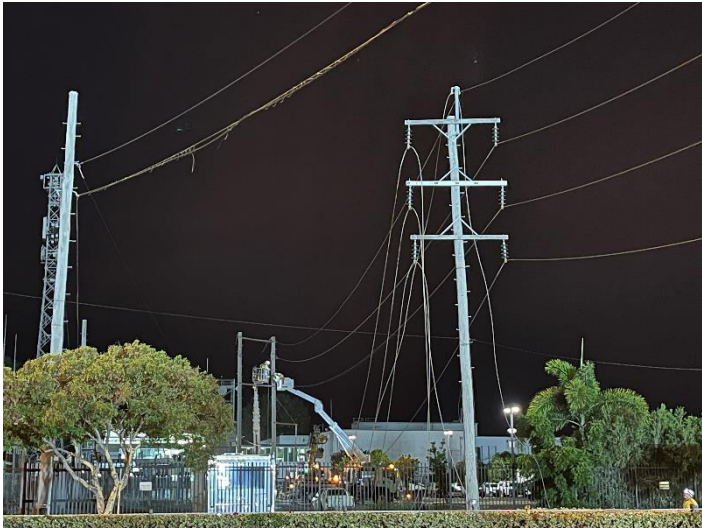
Fig 8 – The powerlines connected to the old substation are lowered to the ground and removed.
