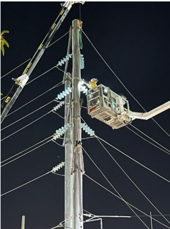
Fig 5 – Each of the powerlines are carefully disconnected from the overhead network at the pole.
