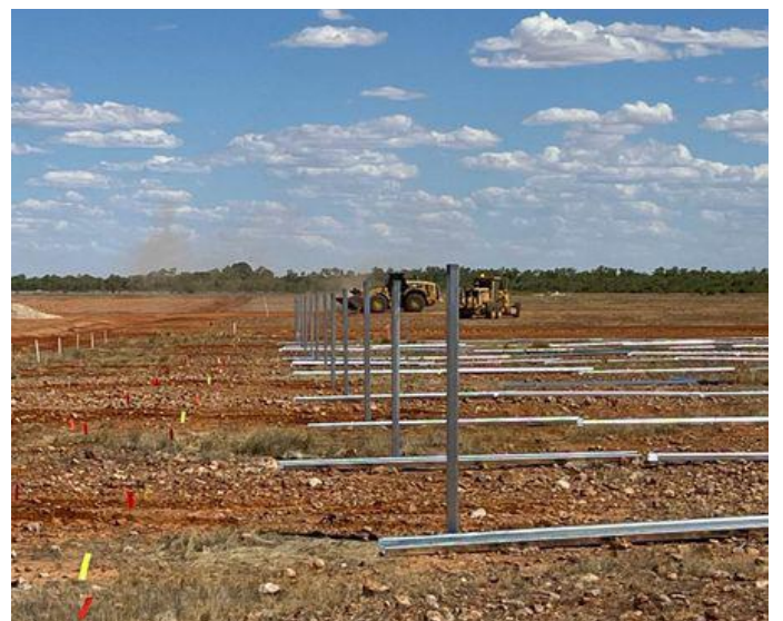
Fig 3 – Civil work and construction of the solar array is happening concurrently on site, with good progress is being made.
