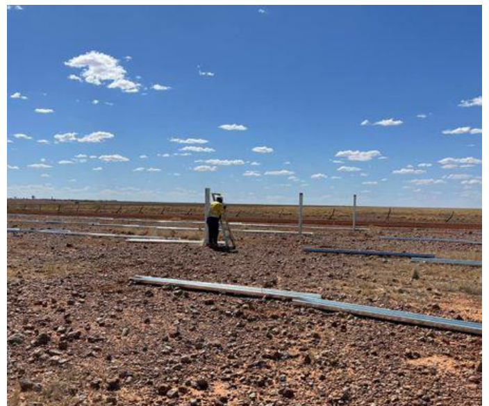
Fig 2 – Delivering a quality job - the team ensures the posts are straight and aligned before starting the framing work.
