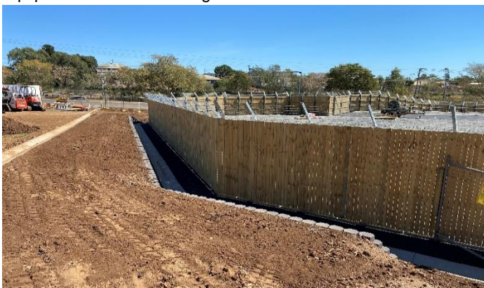
Fig 2 – Security fencing is installed around the substation.
