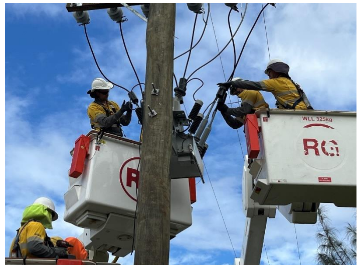
Fig 5 – It was all hands on deck as the overhead crews installed a new high-voltage pole and gas switch at Alligator Creek.
