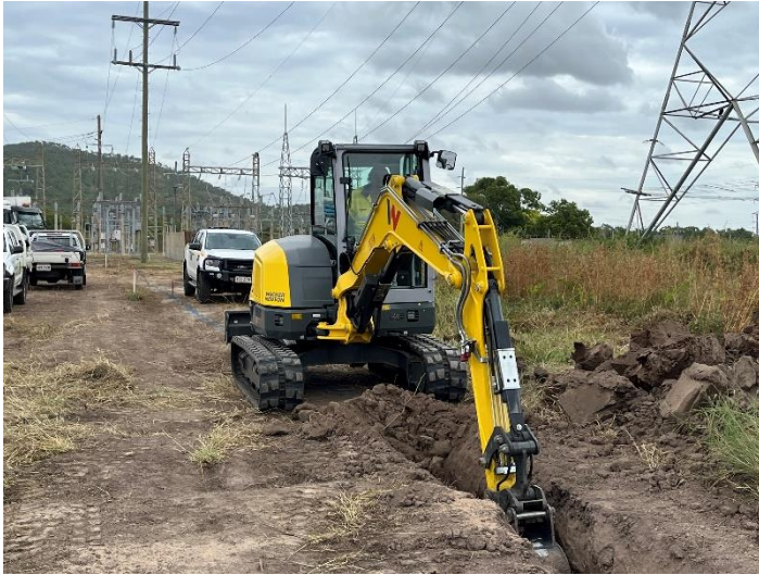
Fig 3 – Excavation of trenches where conduits are being installed to house the underground cables.
