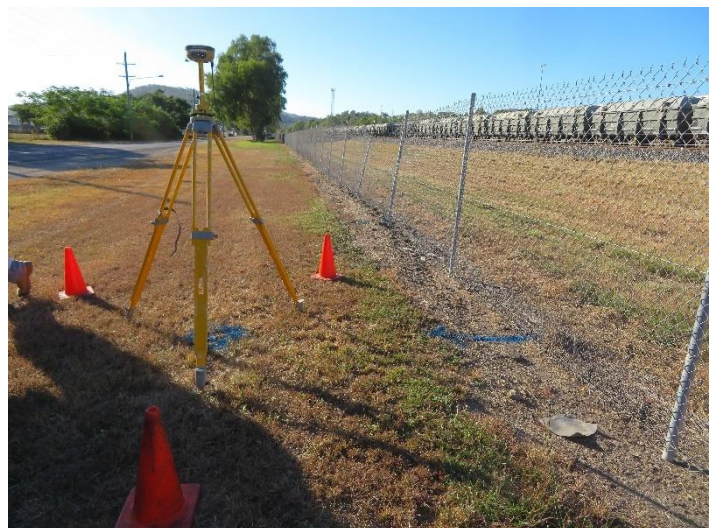
Fig 2- Surveying the area to identify existing assets and map the locations for the new cables.
