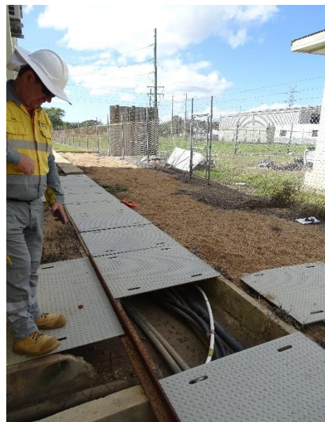
Fig 1- The project manager inspects the old cables which will be replaced this year as part of the upgrade project.
