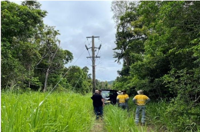
Fig 11 – The project team discuss the location of the new poles in Ergon's easement adjacent to Shute Harbour Rd near the airport.
