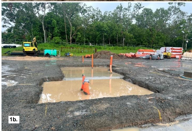
Fig 1a and 1b - heavy rain caused some delays to scheduled work at Cannonvale substation.
