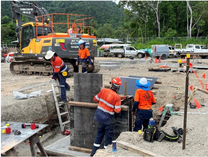
Fig 3 - Contractors prepare concrete formwork in the substation yard for the electrical equipment foundations.
