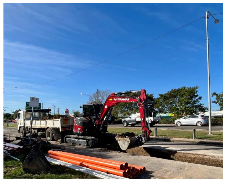
Fig 2 – Excavation along Woolcock Street Service Road for the installation of electrical conduits which will house the new 66kV cable.
