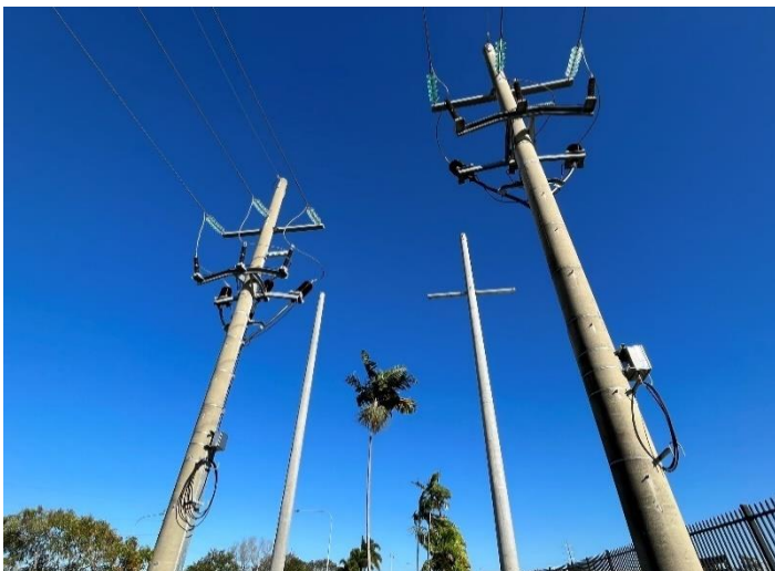
Fig 8 – New concrete poles behind Townsville City Council Depot ready for cable to be pulled and connected to the overhead network.
