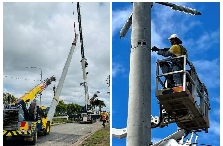
Fig 6 – Two new concrete poles are installed behind Garbutt substation. Ergon overhead field worker bolts the two halves of the 26-metre pole together.
