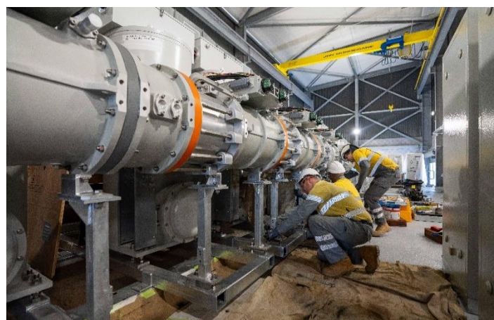
Fig 1 – A look inside the new Garbutt substation building where Ergon's specialist substation crew is installing the GIS.
