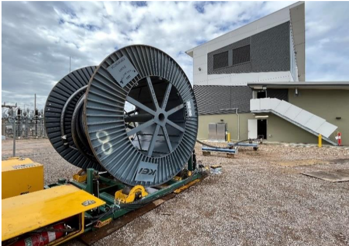
Fig 5 – The new 66kV underground cable rolls of a massive cable drum as it's fed into the new substation building.
