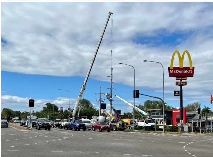
Fig 7 – The top portion of the 25m concrete pole is carefully lifted into place in front of Macca's on Woolcock Street.
