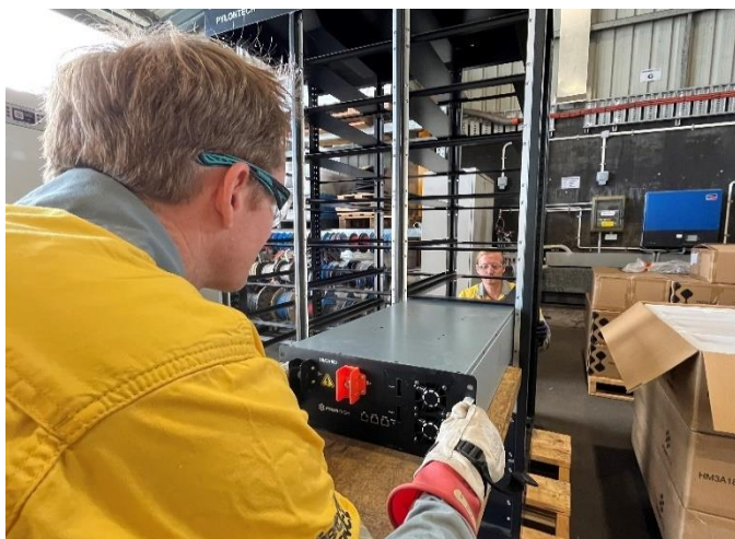
Fig 4 – Dave and Jake are installing the first of the 23 battery units into the battery rack.
