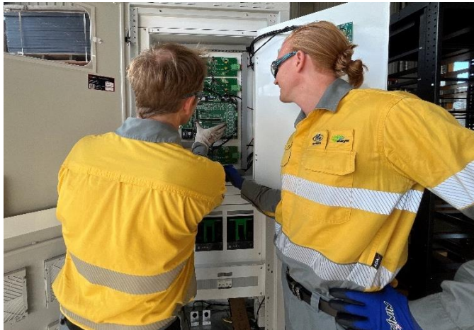
Fig 2 – Jake and Dave from the Fringe of Grid team working on the inverter for the Microgrid Feasibility Study.
