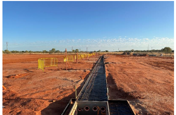
Fig 2 – Installation of conduits for the underground cables that will connect the solar farm to the power station has been completed.
