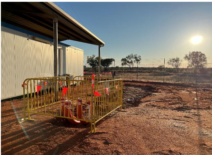
Fig 1 – Installation of conduits for the underground cables that will connect the solar farm to the power station.
