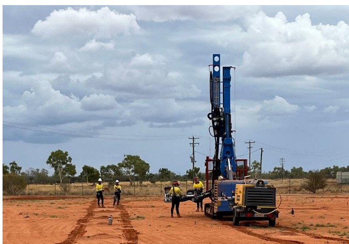
Fig 5 – Crews using the drilling rig to bore hole for the solar array posts.
