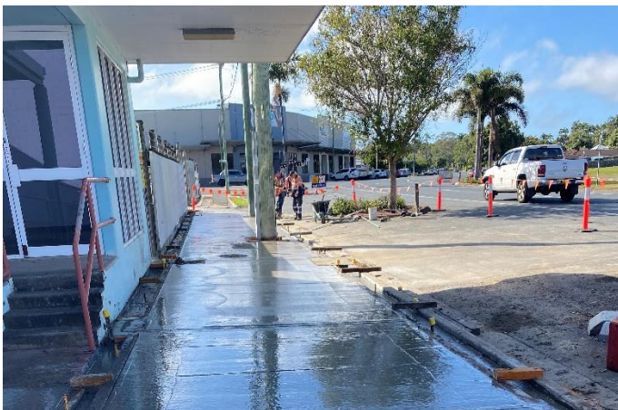
Fig 4 – The new footpath is poured between Watson's Fencing and Inner Labyrinth on Gordon Street.
