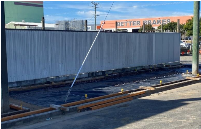
Fig 3 – The area is levelled, and the formwork and reo mesh are installed, ready for pouring the new concrete footpath.
