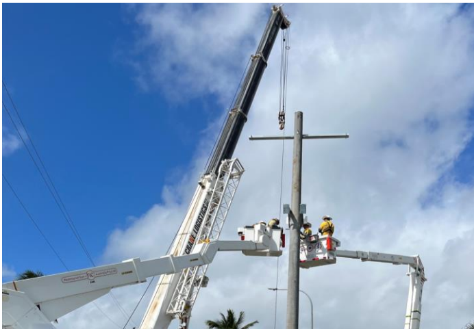
Fig 11 – concrete pole at Jubilee Pocket is craned into place and Ergon crews attach crossarms and other equipment ready for the powerline to be strung.
