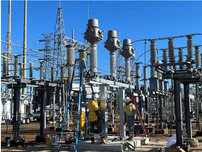
Fig 6 – Ergon crews upgrading equipment at the Proserpine substation as part of the Whitsundays Network Upgrade.
