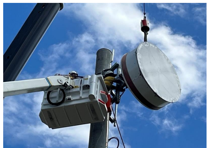
Fig 5 – Communications tower in Proserpine is craned into position and the antenna mounted in place.
