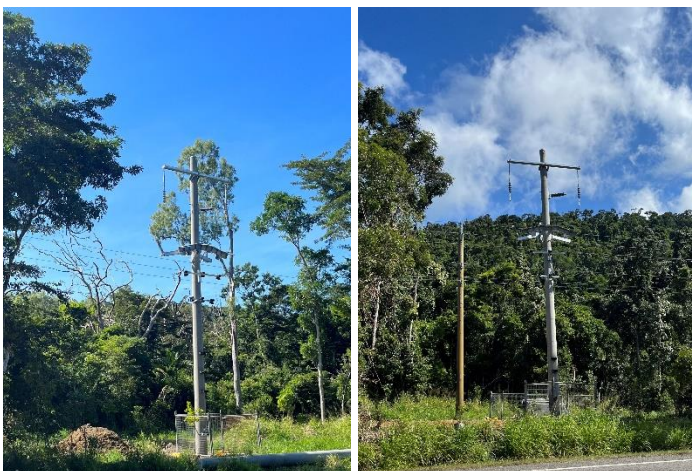
Fig 12 – New poles on the edge of Conway Park at Flametree near Whitsunday Airport.
