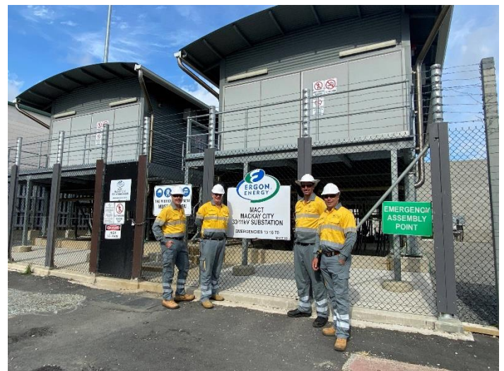
Fig 2 – New Mackay City Substation built to withstand a one in 200-year flood event
