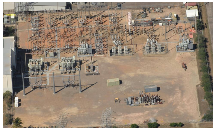
Figure 2 – Old substation equipment will be replaced with modern equipment and removed at the end of project.
