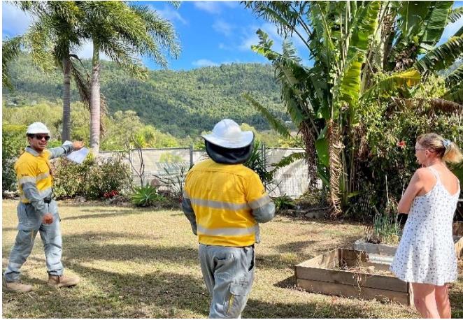
Fig 3 – Ergon project staff discuss the sewer relocation and retaining wall installation with one of our substation neighbours.
