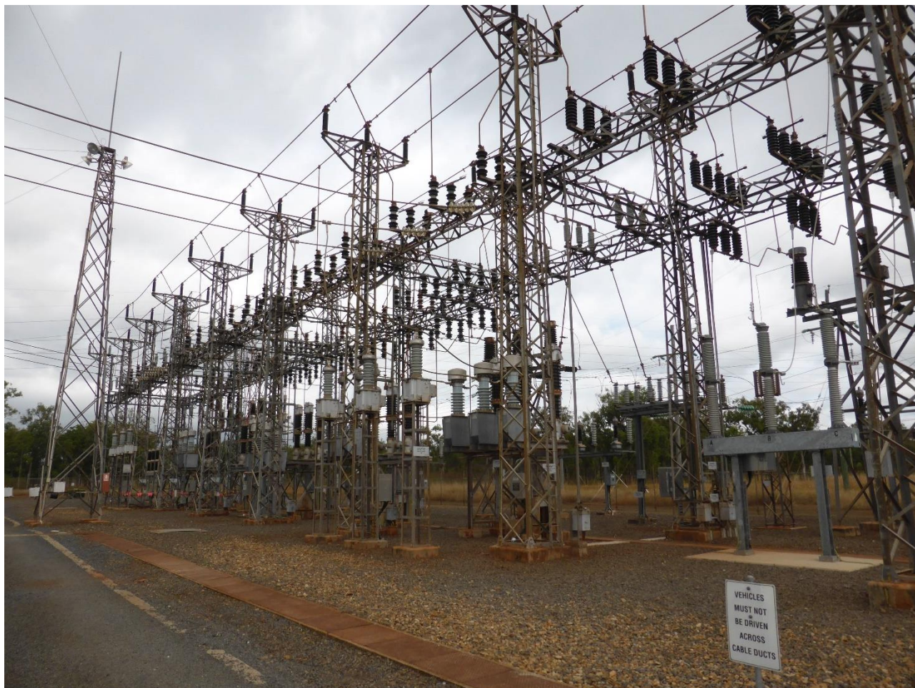
Figure 11: Existing Turkinje bus structure and aged 66kV plant
