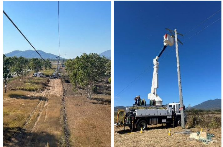
Fig 4- Local overhead crews completing maintenance including replacing crossarms, conductor, insulators, and other hardware.
