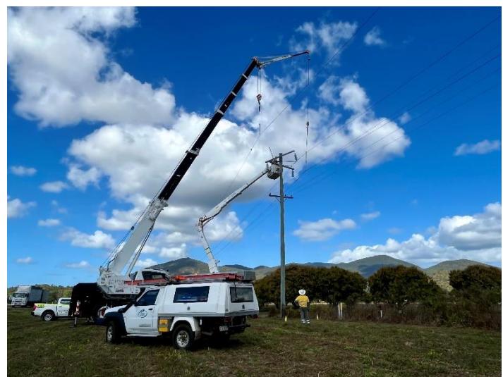
Fig 5 - Bringing in the big guns - a large crane was bought in to lift the live 66,000-volt powerline clear of crews while they replace cross arms at Alligator Creek.
