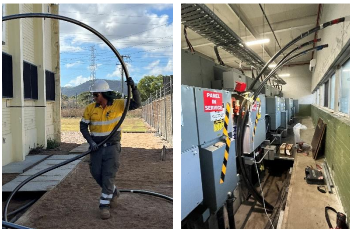
Fig 1 - Our specialist underground crew installing the new cables that connect the substation to the local overhead electricity network.
