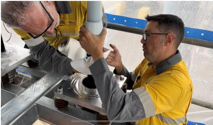
Fig 11 – Behind the scaffold shroud high in the air the team thoroughly strip the cable, remove water blocker material, and reassemble before greasing the polymer cup and slipping it over the cable in preparation for the final components of the termination kit to be installed.
