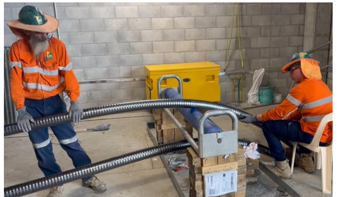
Fig 12 – The 66kV underground cables fed into the substation.
