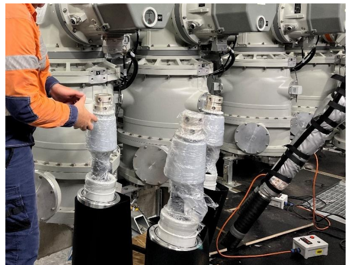
Fig 5 – Termination kits assembled onto each phase which is cleaned (and cleaned again) and wrapped in gladwrap.
