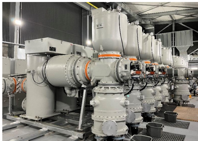
Fig 1 – The transformation inside the Garbutt substation building - the first high voltage cables have been run and the GIS installed.
