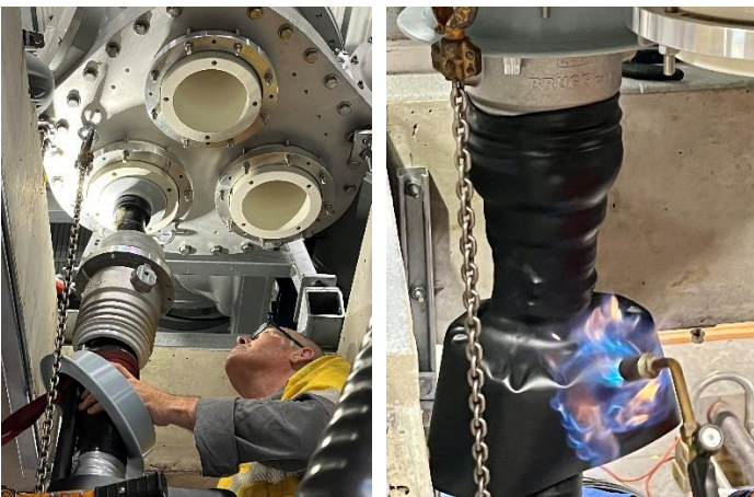
Fig 8 - One by one the phases are manoeuvred into place in the pots and connected to the GIS. Then heat is applied to the heat wrap sealing the termination.
