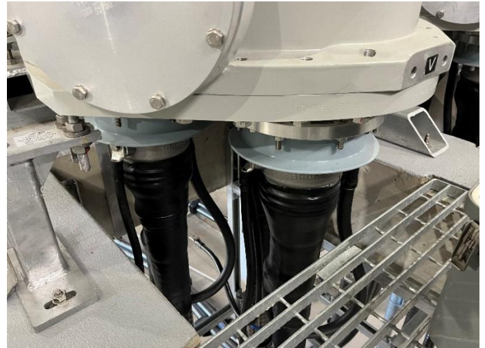
Fig 9 – The three phases of a 66kV feeder connected to the GIS.
