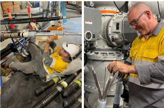
Fig 4 – Each wire in the conductor is meticulously separated, water block removed, cleaned, and reassembled.
