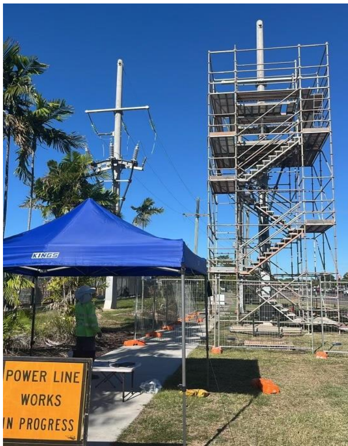
Fig 1 – The scaffolding goes up for crews to terminate and connect the Hermit Park 66,000-volt cable to the network.
