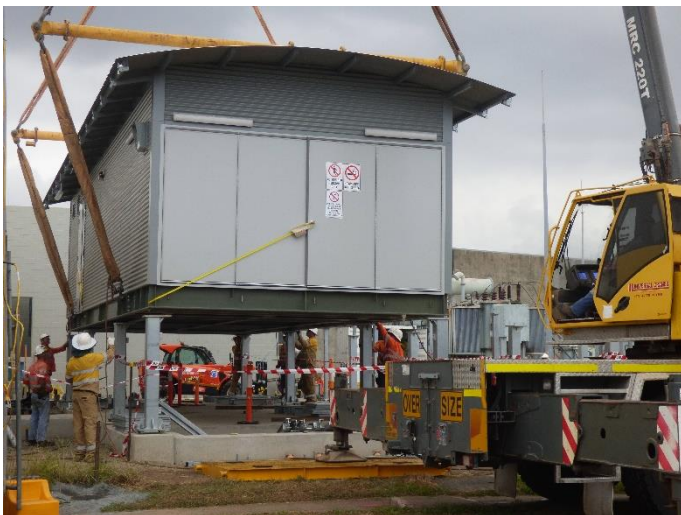
Fig 4 – Building No 1 is manoeuvred into place next to live operational substation and secured onto the steel foundations.
